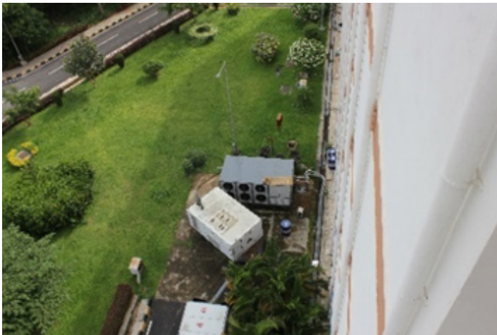
Ground Cooling facility
